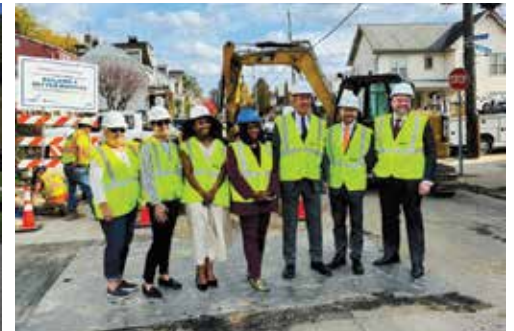
I joined local and federal leaders to celebrate Pittsburgh Water & Sewer Authority's work in replacing over 20,000 lead service lines and an ambitious $1.8 billion plan to remove even more.
