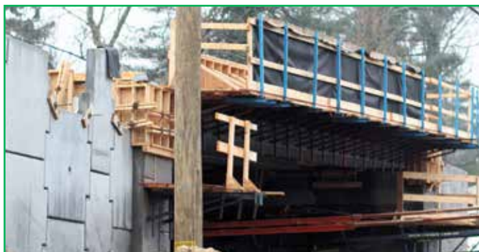
Construction on the College Avenue bridge at Haverford Avenue in Haverford Township is expected to be completed by late May, according to PennDOT.
