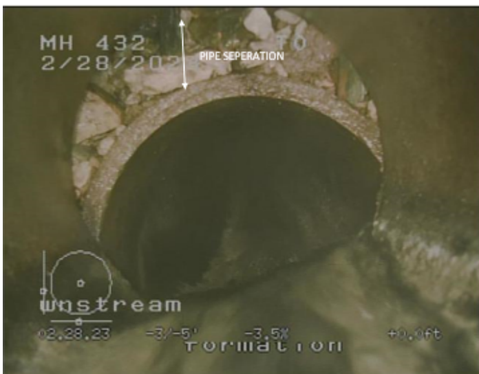
Photo 3. Camera view inside an active sewer pipe in East Whiteland, Chester County shows pipeline break which allows raw sewage to enter the environment.
