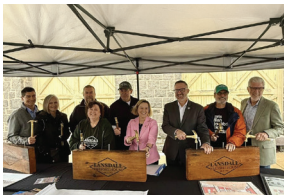
I was honored to celebrate the groundbreaking of Lansdale Freight House with Discover Lansdale .
