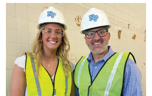
Breaking tile to kick off the renovations of the North Penn High School pool.
